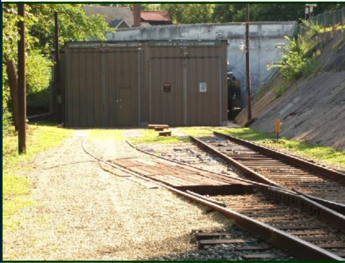
This photo shows the new “crossing” over the Isaacs car barn maintenance barn lead track. Now delivery trucks and automobiles can cross over the rails and snuggle right up to the car barn door without tearing up a tire or two. ( John Prestholdt photo )
